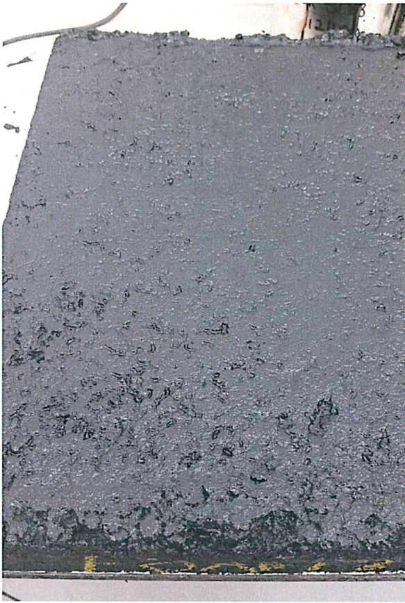
Figure 2-4: Slab after application of Formulation 3
